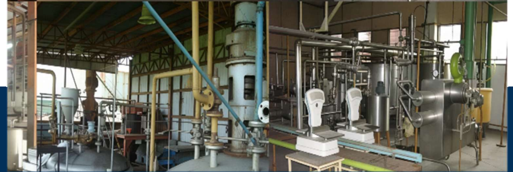
Oil Refining and Fat Modification
